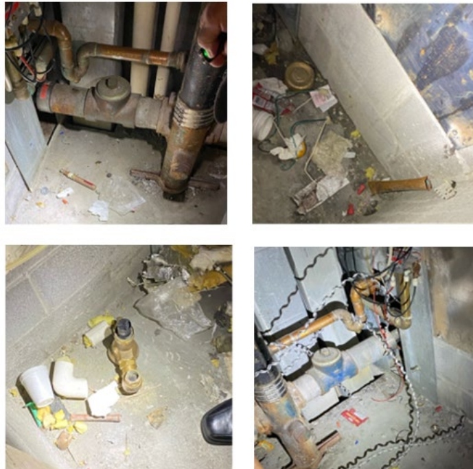
Unsecured pipe chases in the Jail
