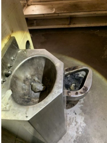
Toilet and sink unit in a cell
